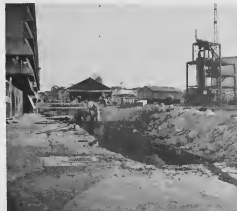
BOTH TANKS and lines were built and installed for Ethyl by the Curacao Drydock Company and subcontractors. Even though the lead compound is almost twice as heavy as water, regular three-inch lines carry the compound to weigh tanks.
